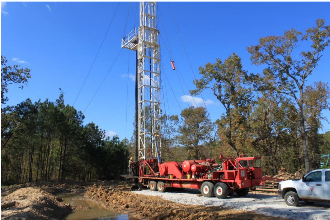
A work over rig running production tubing on the Jack Allen No.7 well
