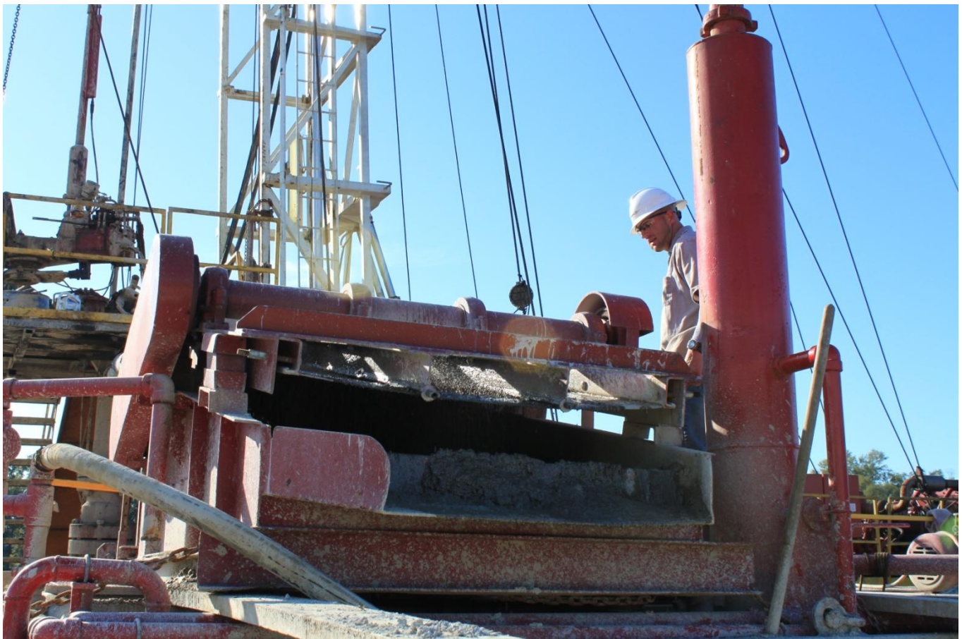
Cement cuttings from the third and final cement plug in the HM Brian No.1 well passing over the shale shakers
