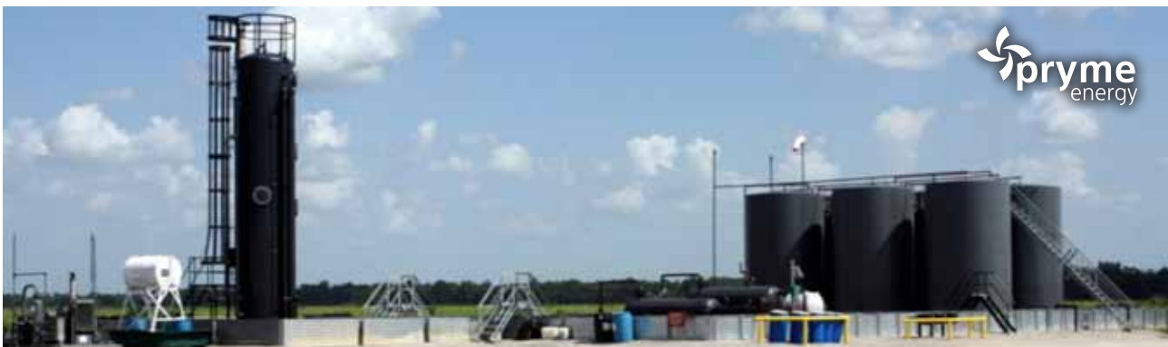
Production facilities at Turner Bayou
