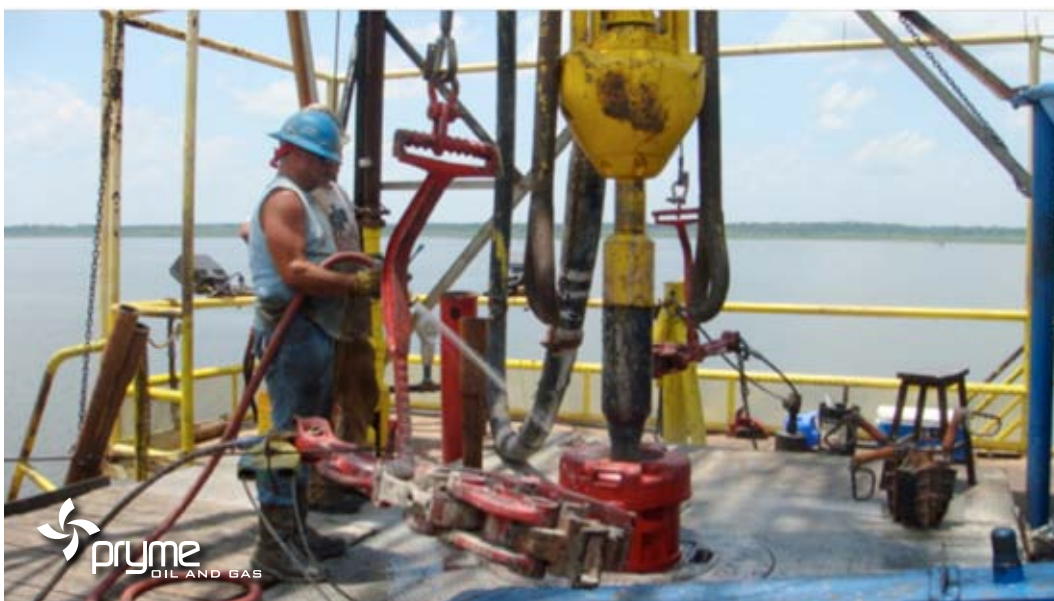
Drilling crews working on the barge mounted rig in Catahoula Lake, Louisiana
