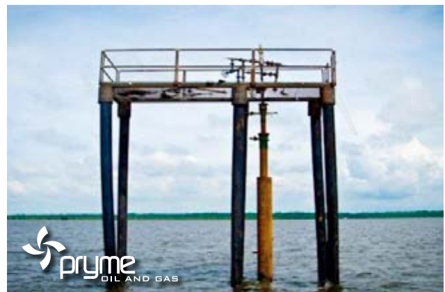
Production platform of the SL 502 No.1 in Catahoula Lake, Louisiana
