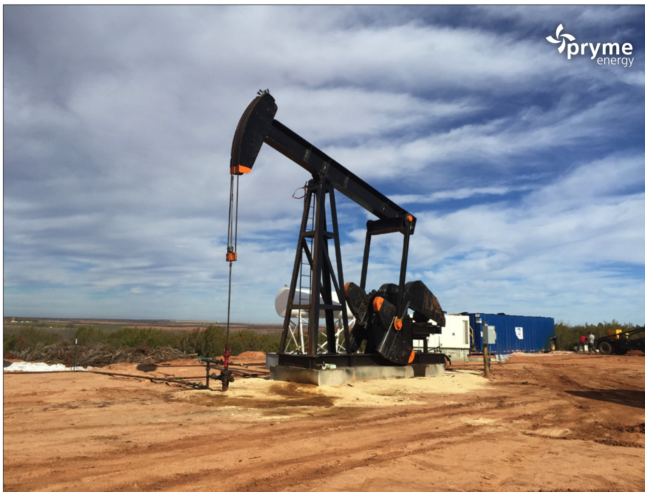
Pumping unit on Mahaffey Bishop well in Capitola Oil Project
