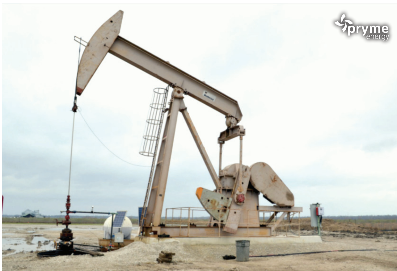
Pumping Unit on Deshotels 13H well
