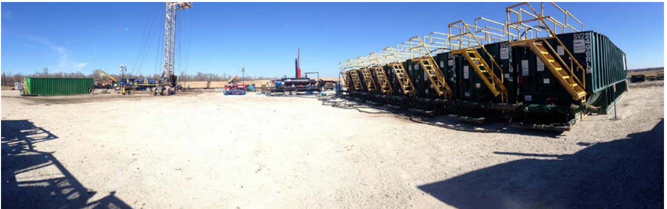
Workover rig running tubing and flow back tanks on Rosewood Plantation 21H well site
