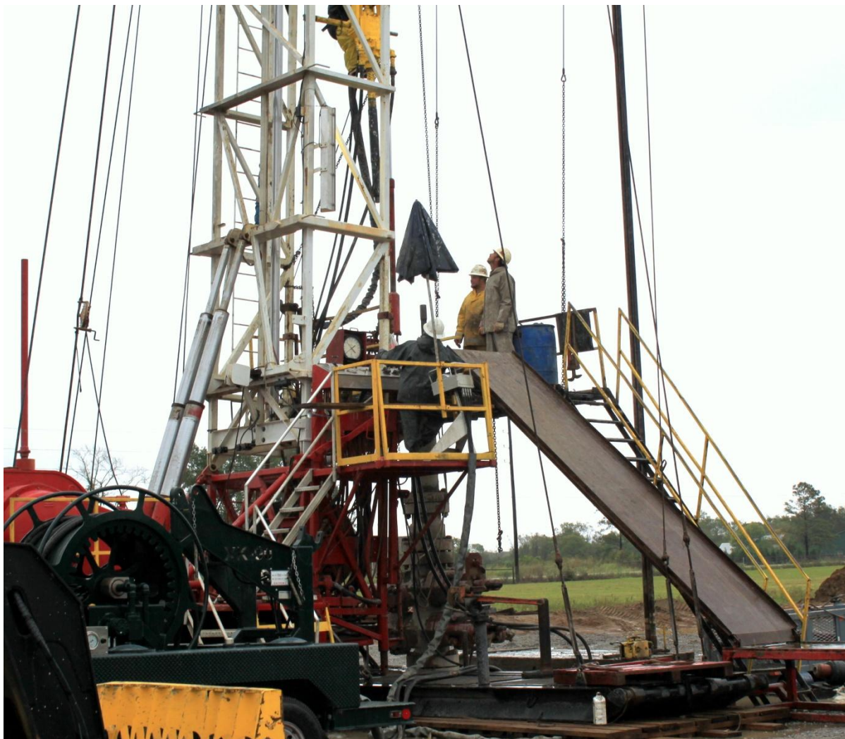
Crews milling through the cast iron bridge piece located at the base of the second cement plug
