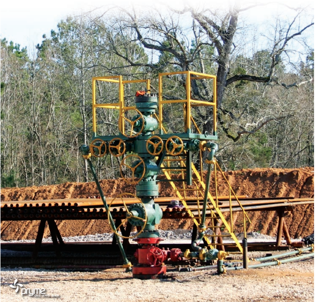
Well head of the Grable 15#1 in the Raven Project
