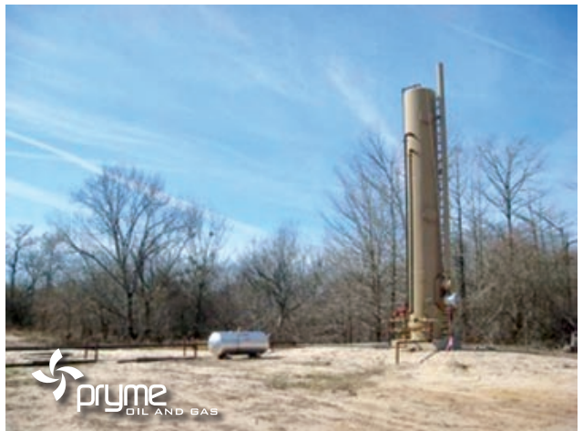
Newly installed production and storage facilities in the Saline Point project
